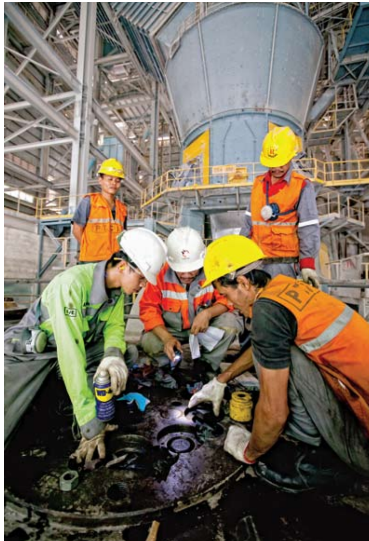
Holcim staff and contractors work on a maintenance job at the Narogong Plant in West Java. Our health and safety standards are the same for both permanent staff and third party employees.
