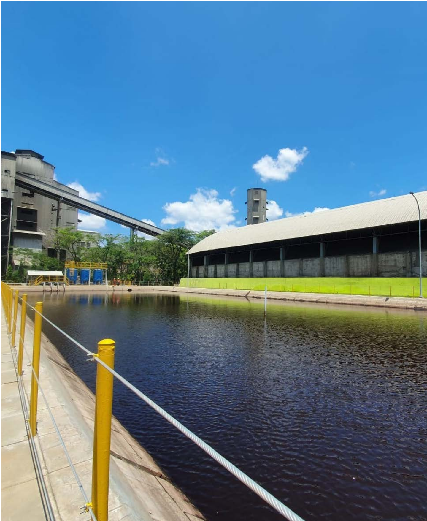
Fasilitas IPAL di Pabrik Narogong. WWTP facility at Narogong Plant.
